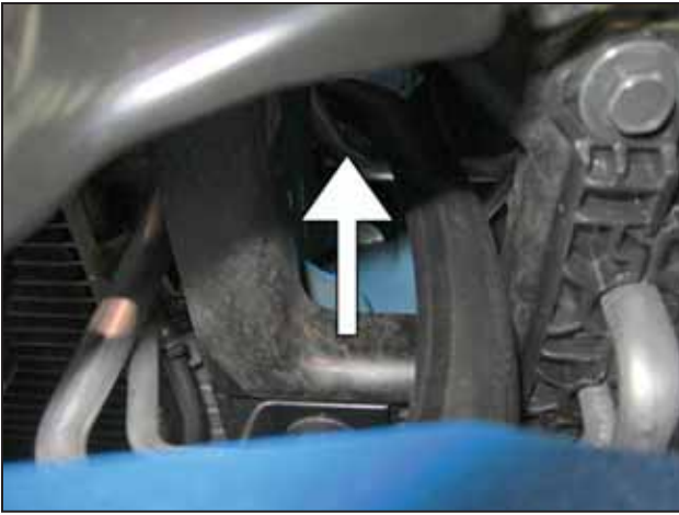
aj. Route the hose up through the area where the OEM inlet duct used to be.
