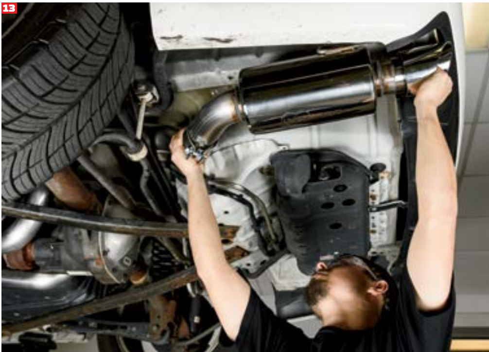
With the 3-inch exhaust tubing in place, Weathers installed the polished, straight-through Hooker mufflers.
