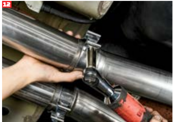
Weathers tightened the clamps slightly to keep all the tubing in place but still allow for adjustment.
