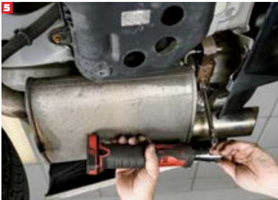
Hooker technician Walker Weathers began our installation by disconnecting the OEM muffler hanger brackets from the chassis.
